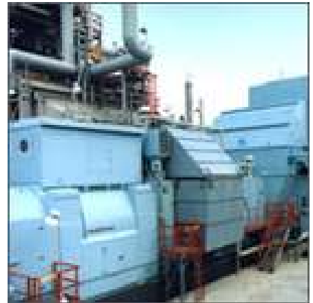
Figure 2: Typical generator cooled with Hydrogen
